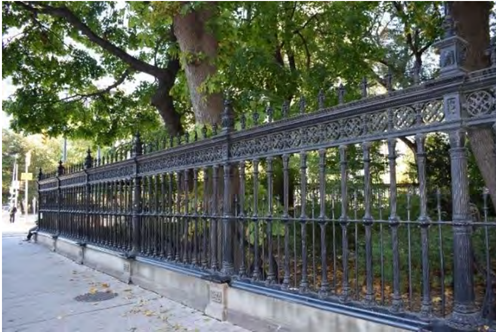
Stone and wrought iron fence on perimeter of the property, facing west
